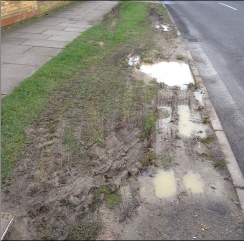
Example of Damage Coneygree Road
